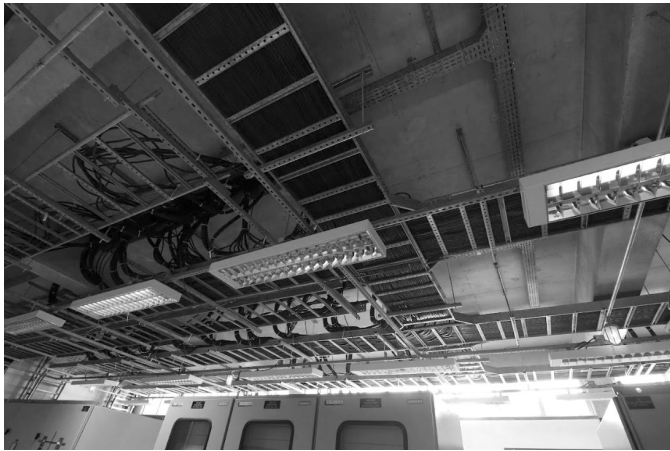
Fig. 1. View of part of the ceiling cable trenches in the control room of Substation ANH.
