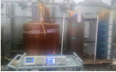
Fig. 4. 15 MVA two-winding transformer.
