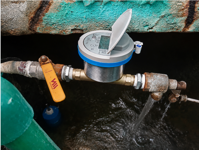
Fig. 2. Installed ultrasonic IoT flow meter at the facility intake.
